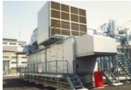
Use of cogeneration facilities greatly reduces emissions of greenhouse gases.
